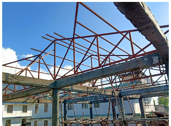
The top floor for our Sidhbari Library is ready for roofing and will become the space for a new study hall
